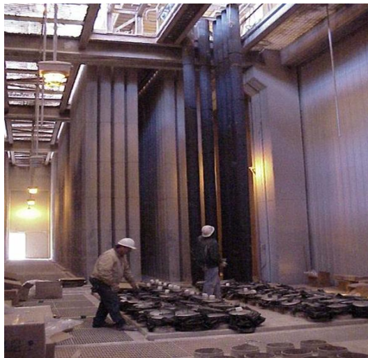
Figure C-2: former GCC baghouse, interior. A GCC employee pushed a cart loaded with emissions sampling equipment through this space to gather data for emissions calculations.
